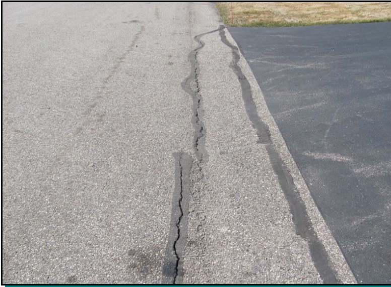
Edge crack and previous crack repair at asphalt street
