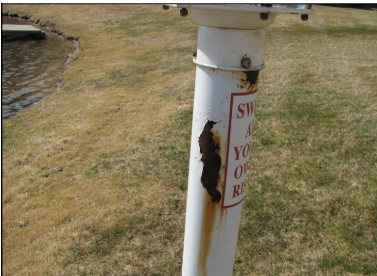
Light pole finish deterioration
