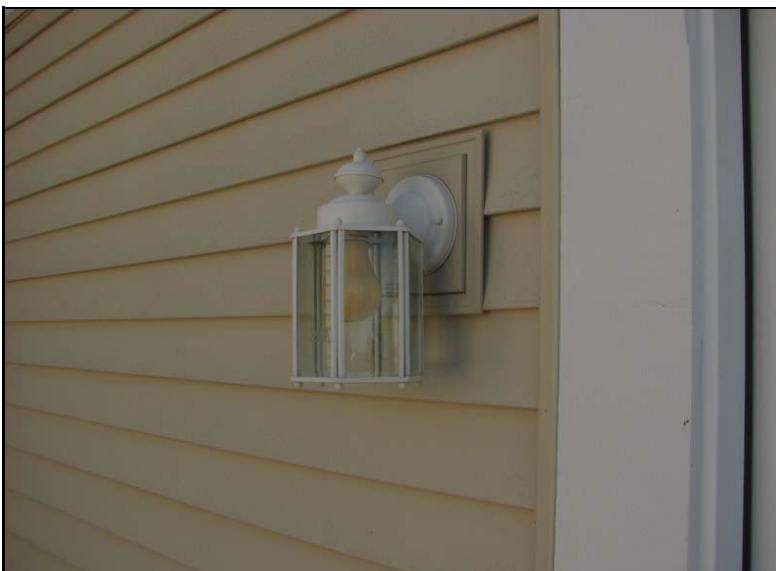
Light fixture at garage service door
