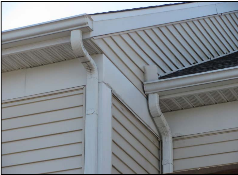
Gutter and downspout assembly, note kick-out flashing to direct stormwater into gutters
