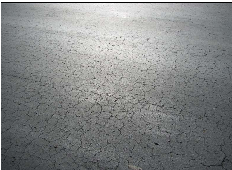
Surface deterioration at driveway
