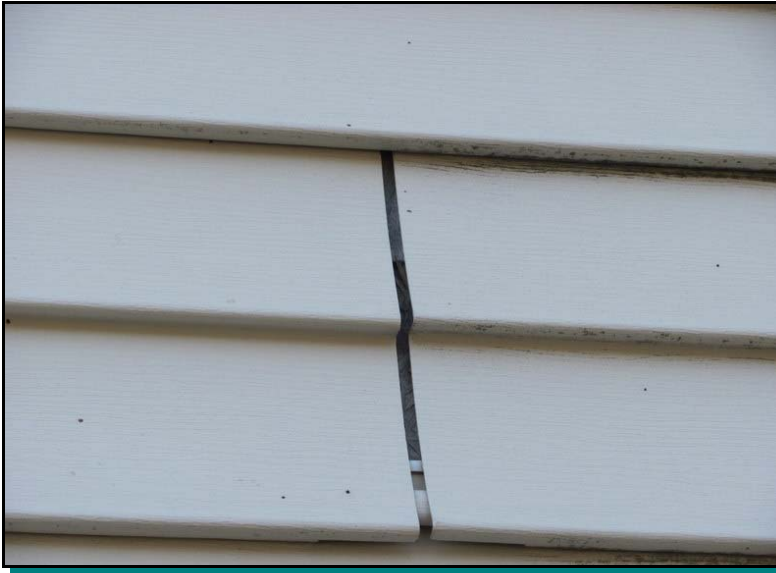
Gap in vinyl siding, note lack of building wrap
