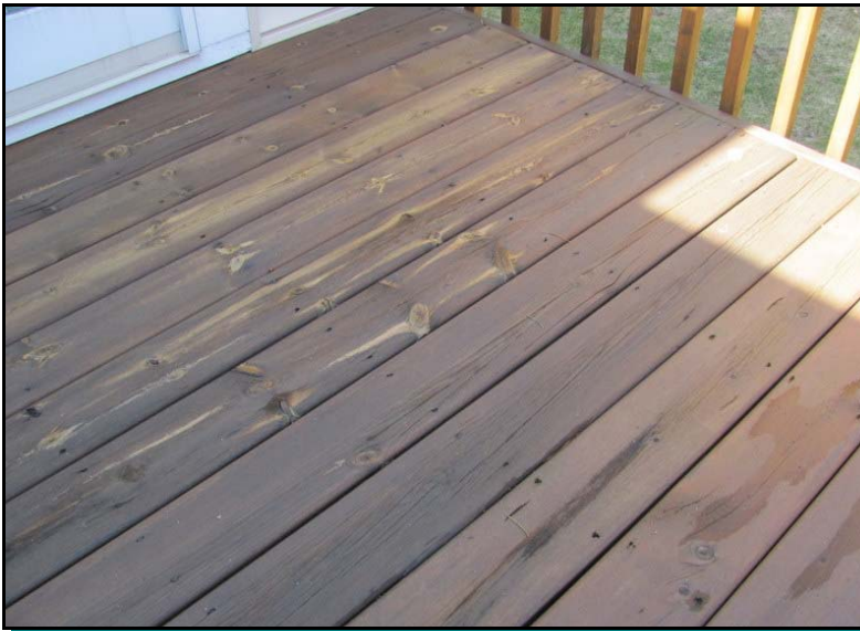
Deck boards, note minor stain deterioration
