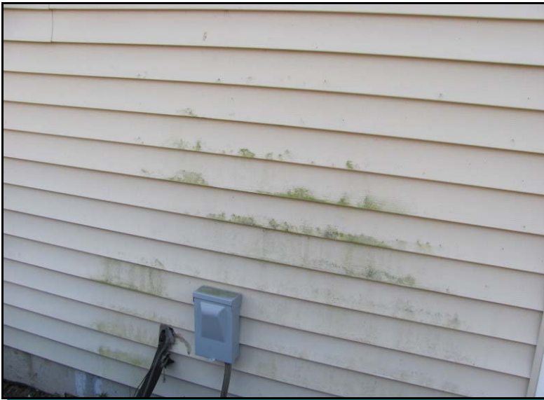
Organic growth at vinyl siding
