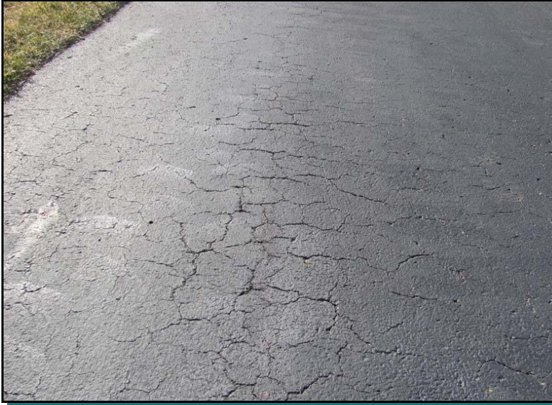
Surface deterioration and developing fatigue cracks at asphalt driveway
