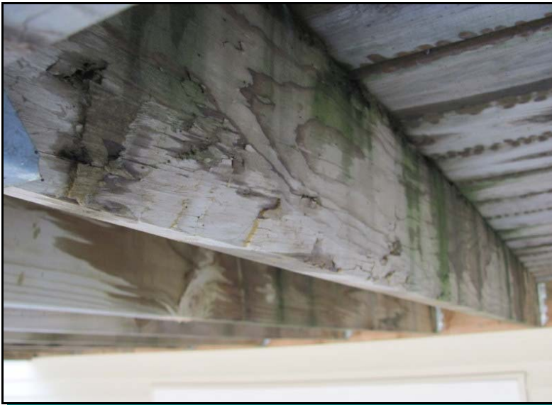
Minor deterioration at balcony joist
